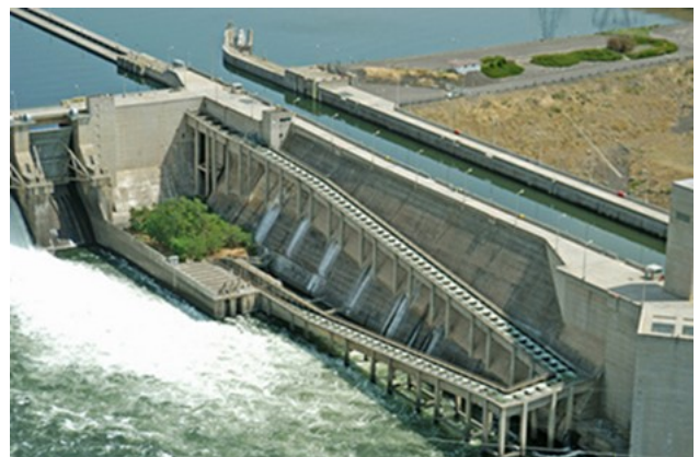
This fish ladder on the Lower Monumental dam on the Columbia River is designed to minimise the impact on migratory fish.
